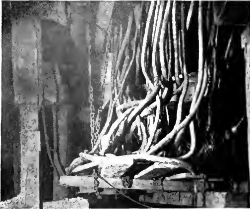
FIG. 2.—EXCAVATION AT ANN STREET, NEAR SCENE OF FIRE.
